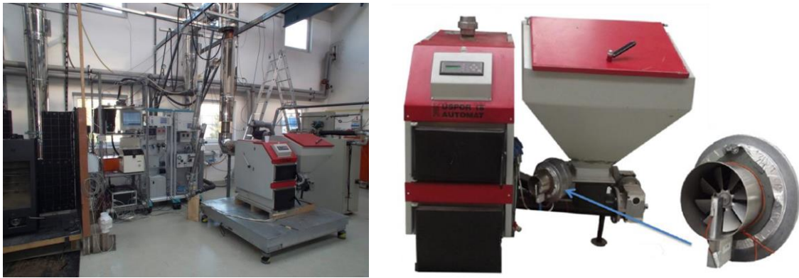
Fig. 1 experimental measurements of pellet boiler.
